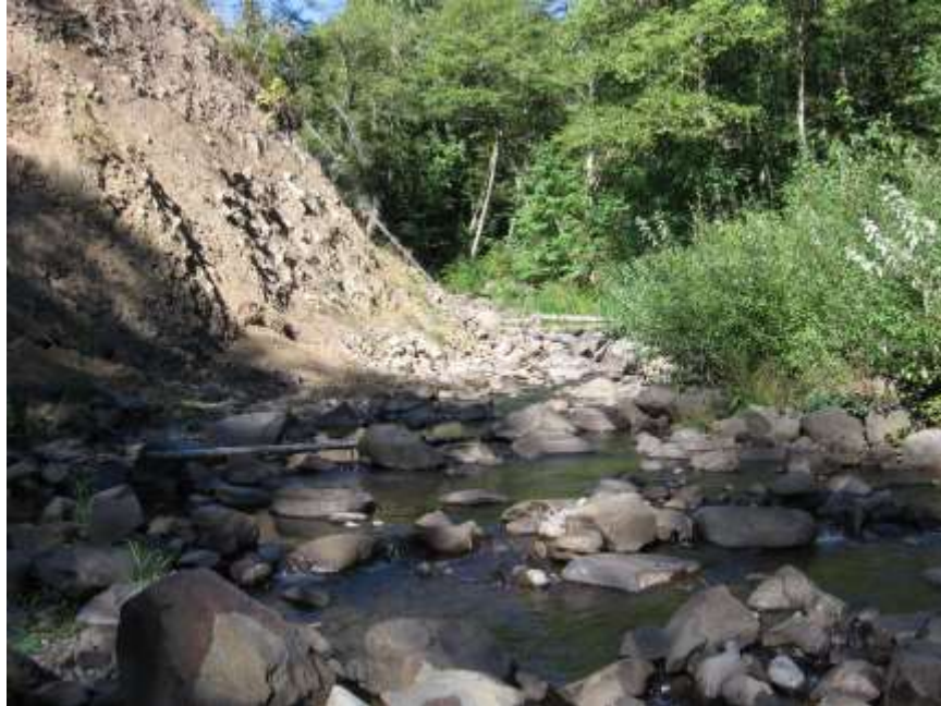
Figure 12 Eroding Bank Near Downstream End of Reach 4
